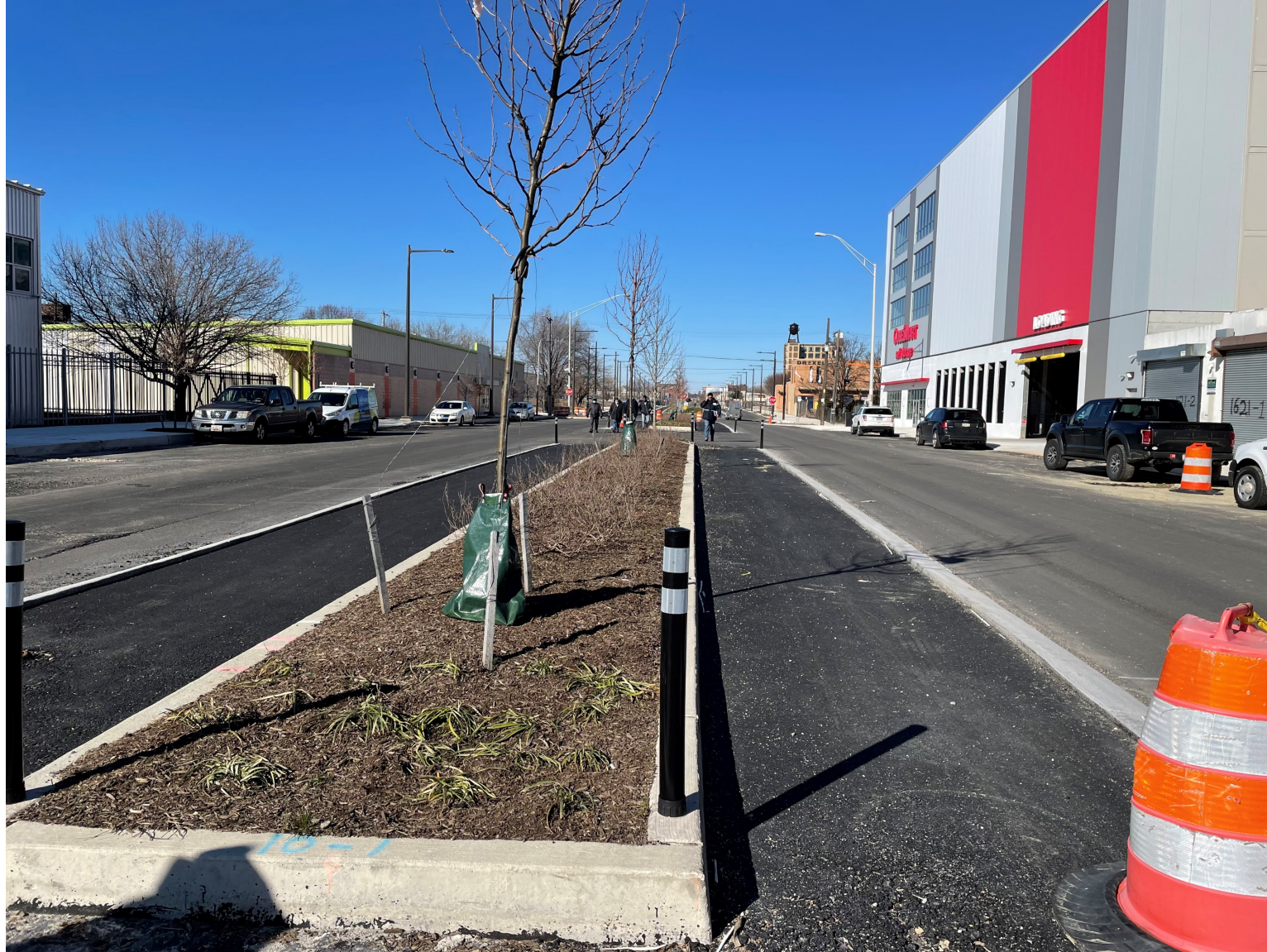
bioswales, trenches, bumpouts
