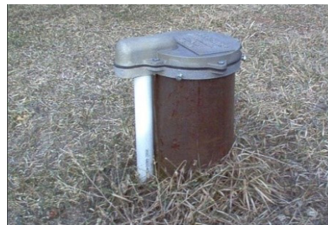
Typical well head in found in yard
