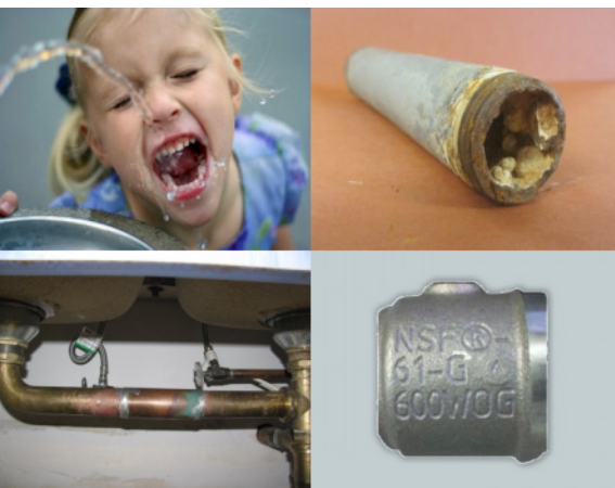
Household plumbing may involve lead-containing components
