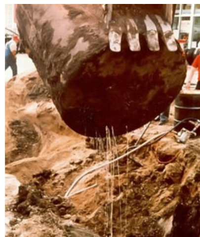
LUSTs can cause significant contamination
