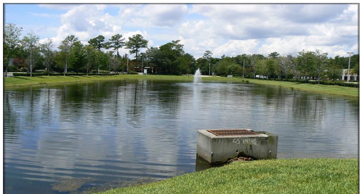
Stormwater pipes often lead to retention ponds before release into our waterways
